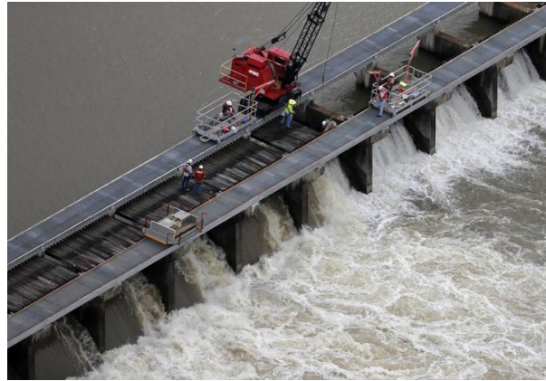
Workers open bays of the Bonnet Carre Spillway, to divert rising water from the Mississippi River to Lake Pontchartrain, upriver from New Orleans, in Norco, La., Friday, May 10, 2019. Torrential rains in Louisiana brought such a rapid rise on the river that the Army Corps of Engineers is opening the major spillway four days earlier than planned. Spokesman Ricky Boyett says the river rose six inches in 24 hours, with more rain expected through the weekend. (AP Photo/Gerald Herbert)
